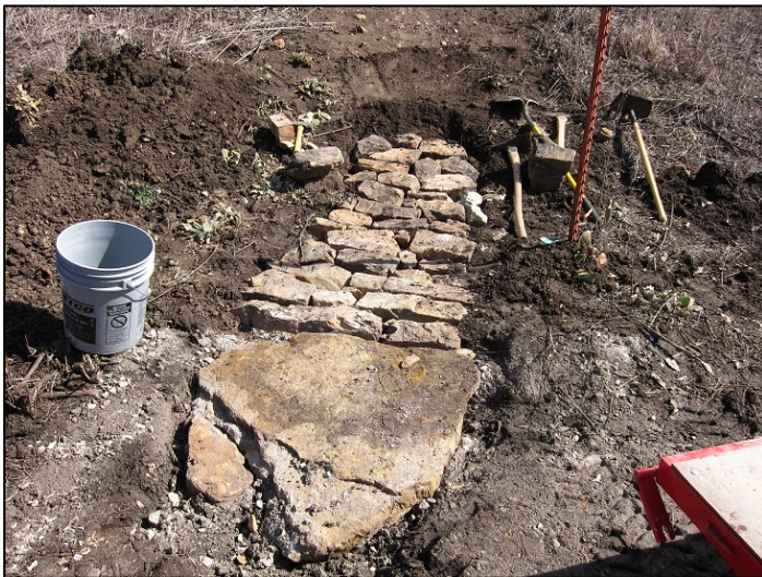
Large Anchor Rock at the Bottom
